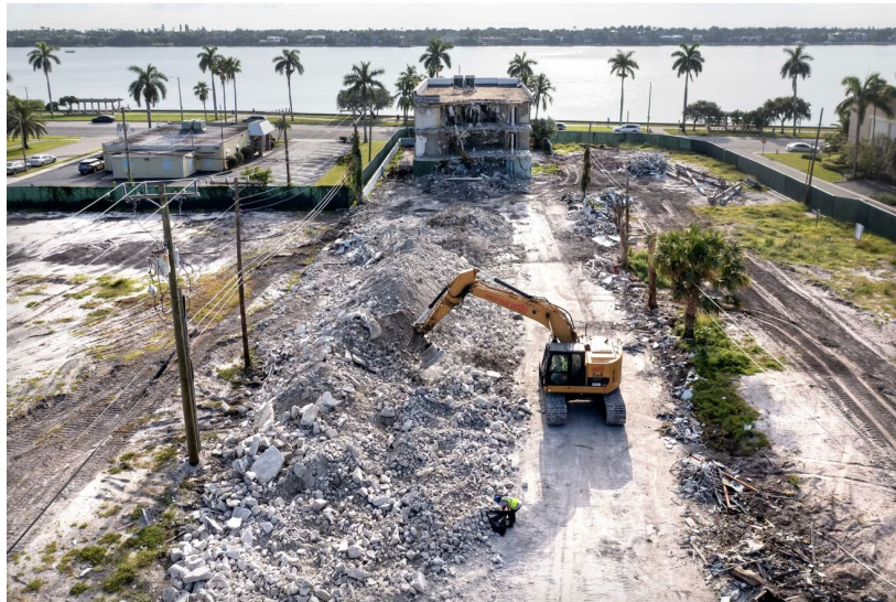
The future home of Olara, a 26-story tower featuring 275 condominiums as part of a mixed-use project at 1919 N. Flagler Drive in West Palm Beach, Florida on September 7, 2023. Greg Lovett, GREG LOVETT/THE PALM BEACH POST
